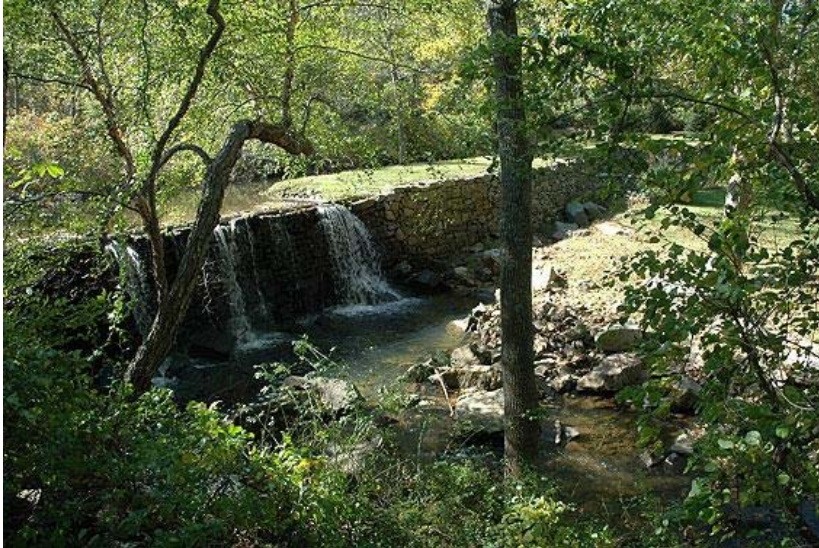
A milldam on Pickering Creek in Chester County, Pennsylvania. The dam spans the entire valley, and is filled to the brim with sediment. (Image: Robert Walter and Dorothy Merritts)
